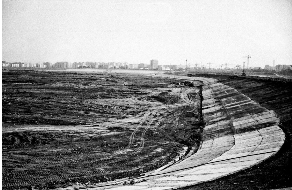
Figure 2.1. A photo of the Văcărești Reservoir in 1989 (Andrei Birsan Vacaresti 1989_web.Jpg (1908×1242), n.d.)
